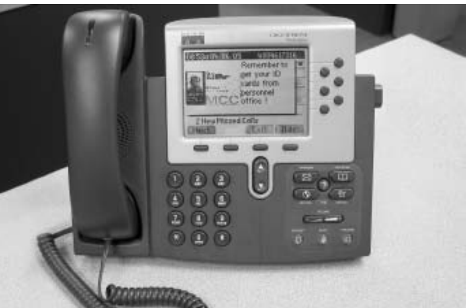
Emergency alerts can be broadcast on CISCO IP phones.
