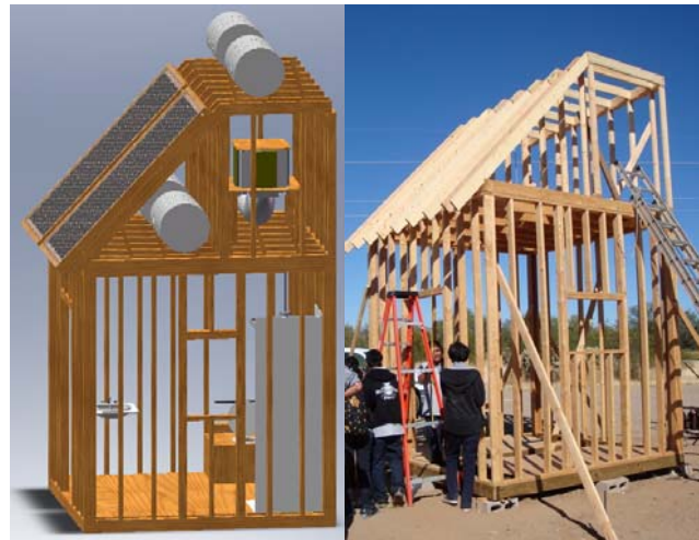
Fig. 3. CAD Drawing of Design (Burns et al., 2008) and Prototype Construction at TOCC, Sells, AZ.
